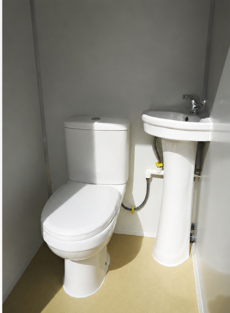
Toilet and hand basin
